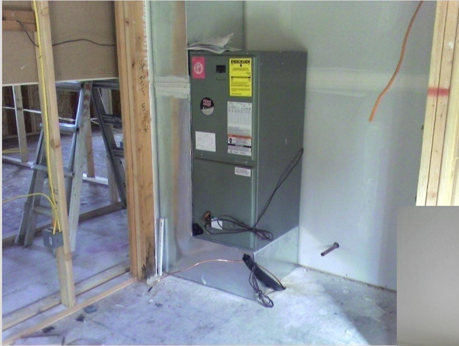
Air Handler Inside
