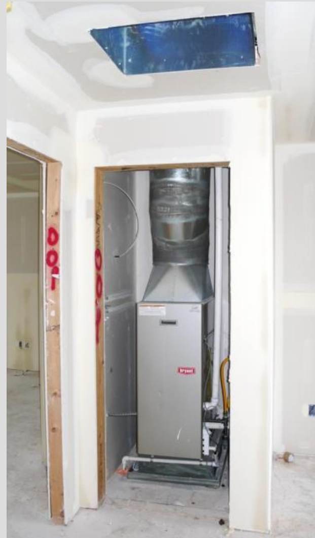
High efficiency furnace inside the structure
