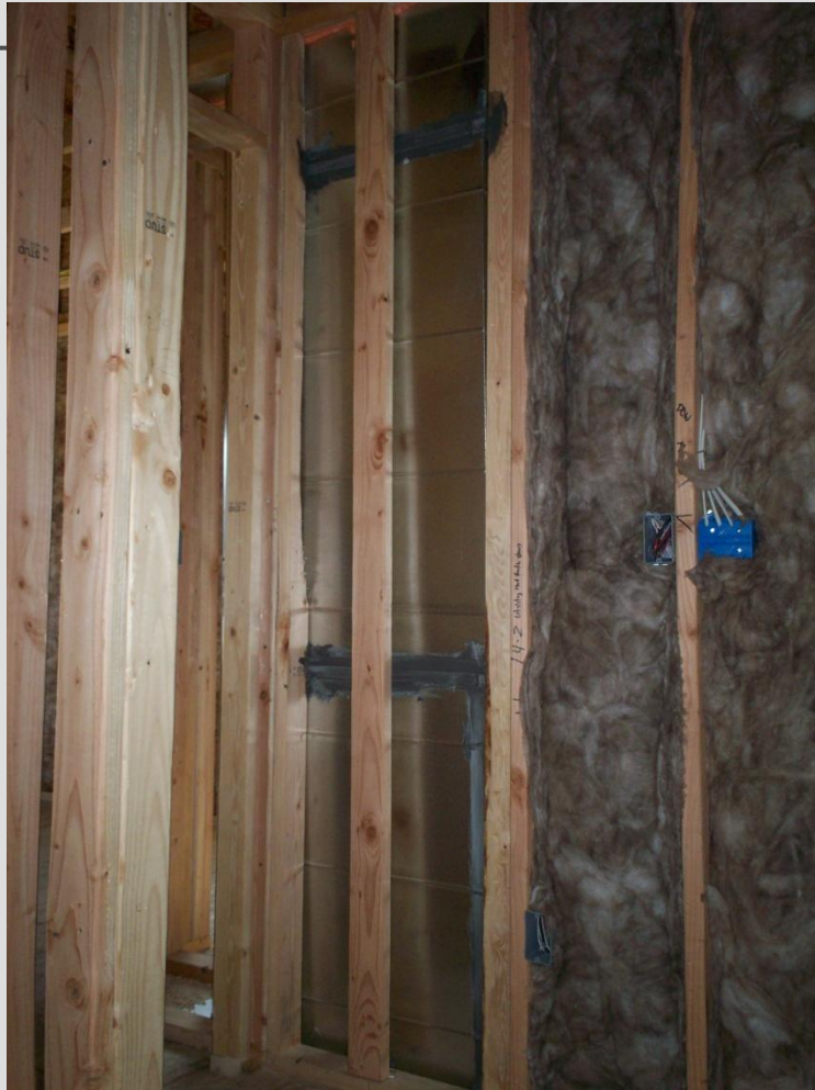
Ducted return inside the house
