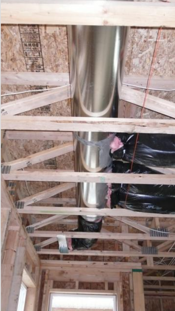
Ducts between floors
