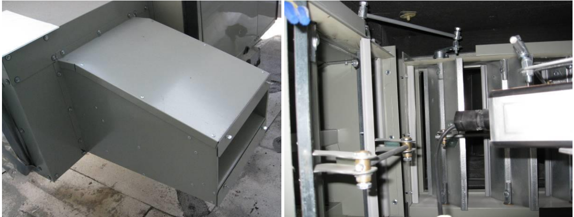
Figure 2: Example of an outside air intake (left) and economizer dampers & actuator (right) for the same small RTU.
